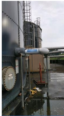
Leachate Holding Tank Line Treatment
